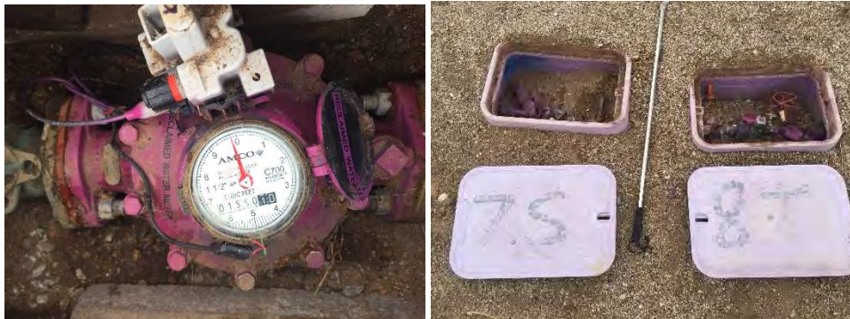
Obtaining flow rates for a tree and a shrub zone (valves on the right) from the dedicated water meter (left).
