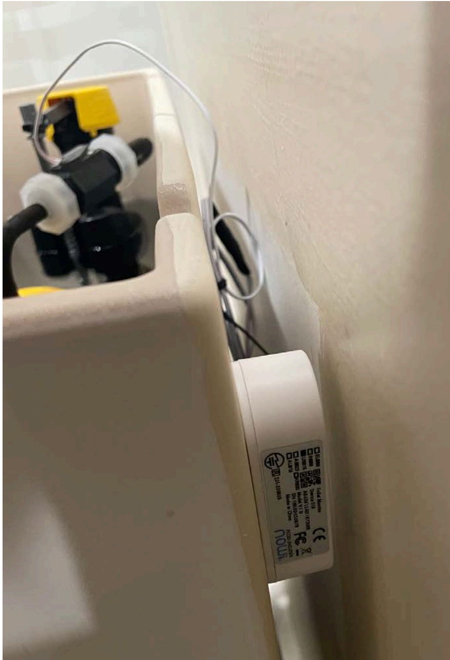
Figure 13- Shows the Toilet Monitor's communication node hidden behind the toilet between the wall.
