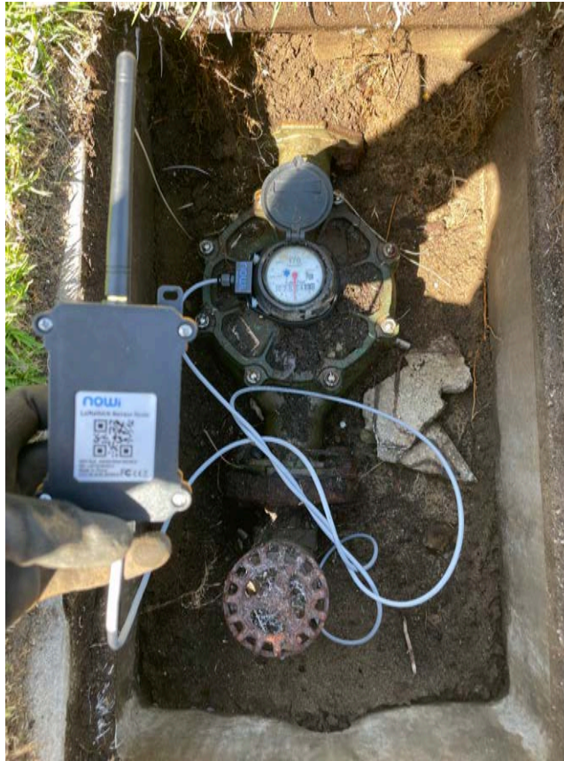
Figure 6 - Is an example installation with the sensor strapped onto the register of a property's water meter.
