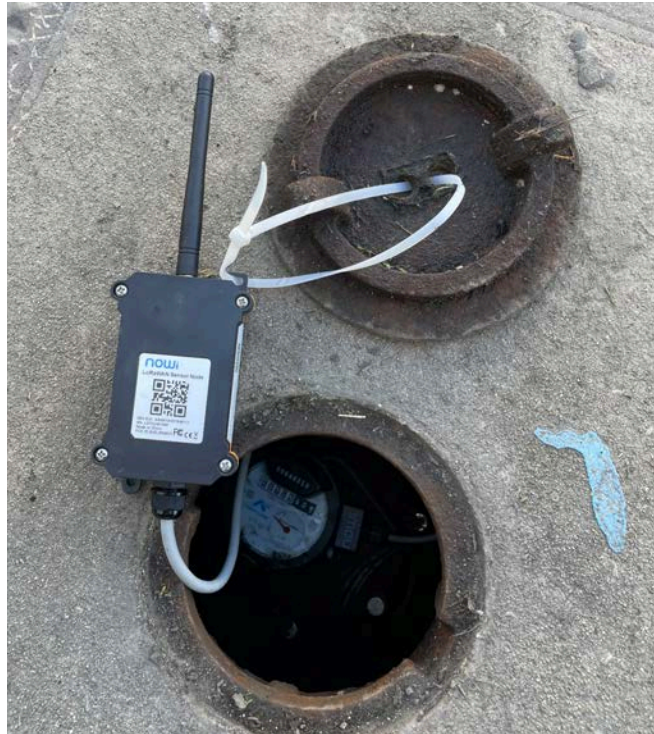
Figure 7 - A building monitor zip-tied to the lid of a water meter pit.
