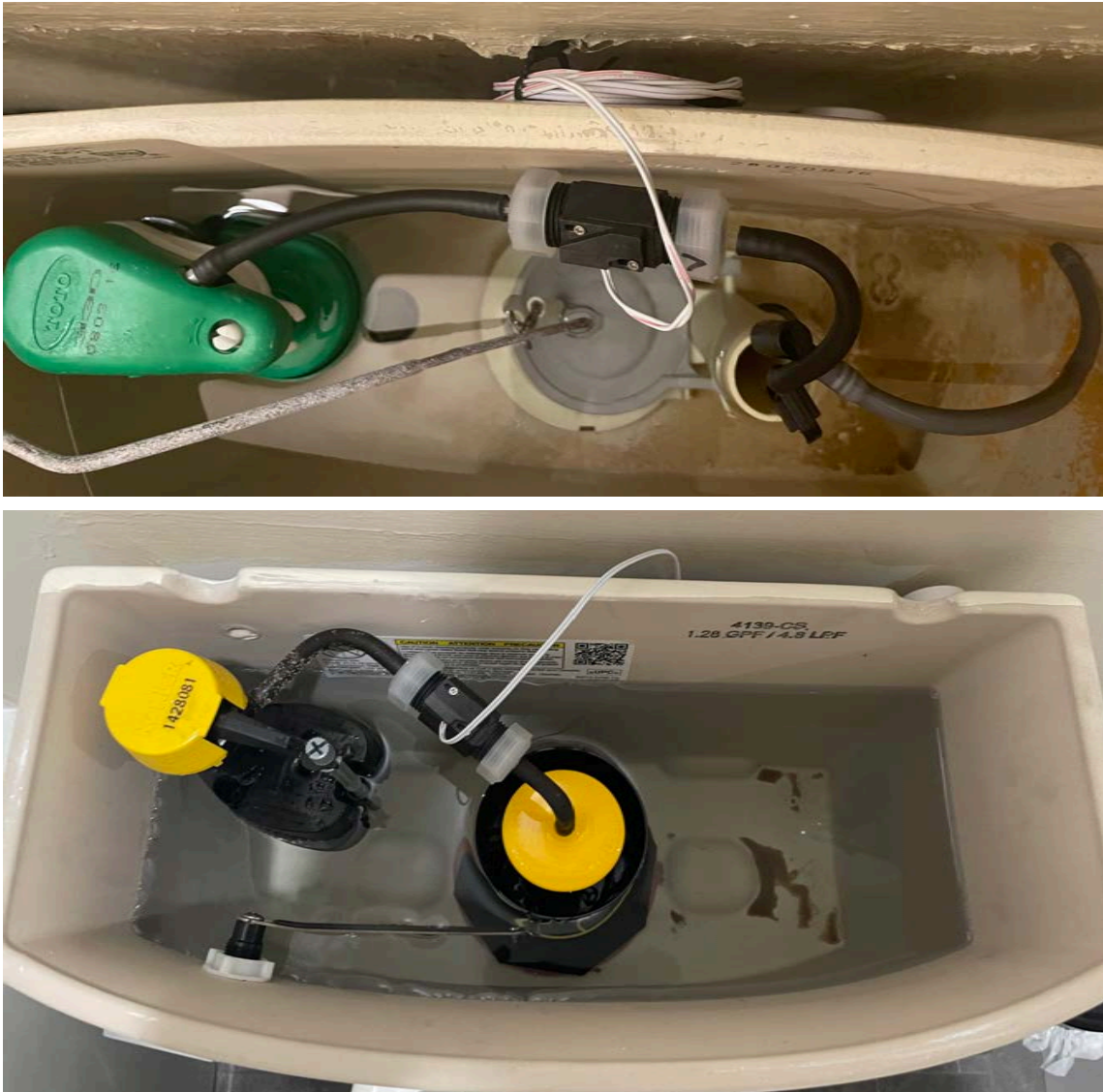
Figure 14 - Shows two examples of how the Toilet Monitor sensor is installed within the toilet.
