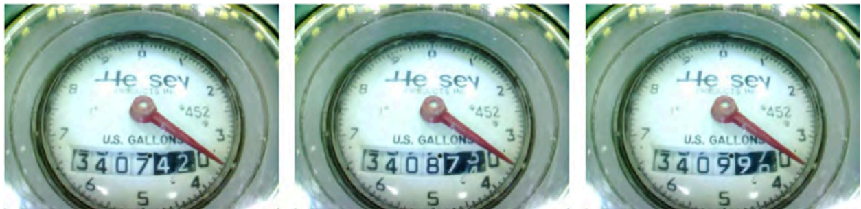
Figure 23 - Consumption numbers changing on the register but the dial is not moving
