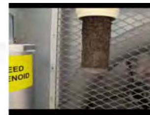
Plugged screen filter prior to blowdown valve
