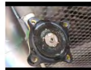
Small amount of debris that passed screen filter that caused valve to stick closed.
