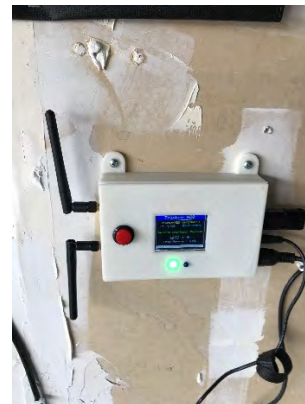
Enclosed circuit boards
