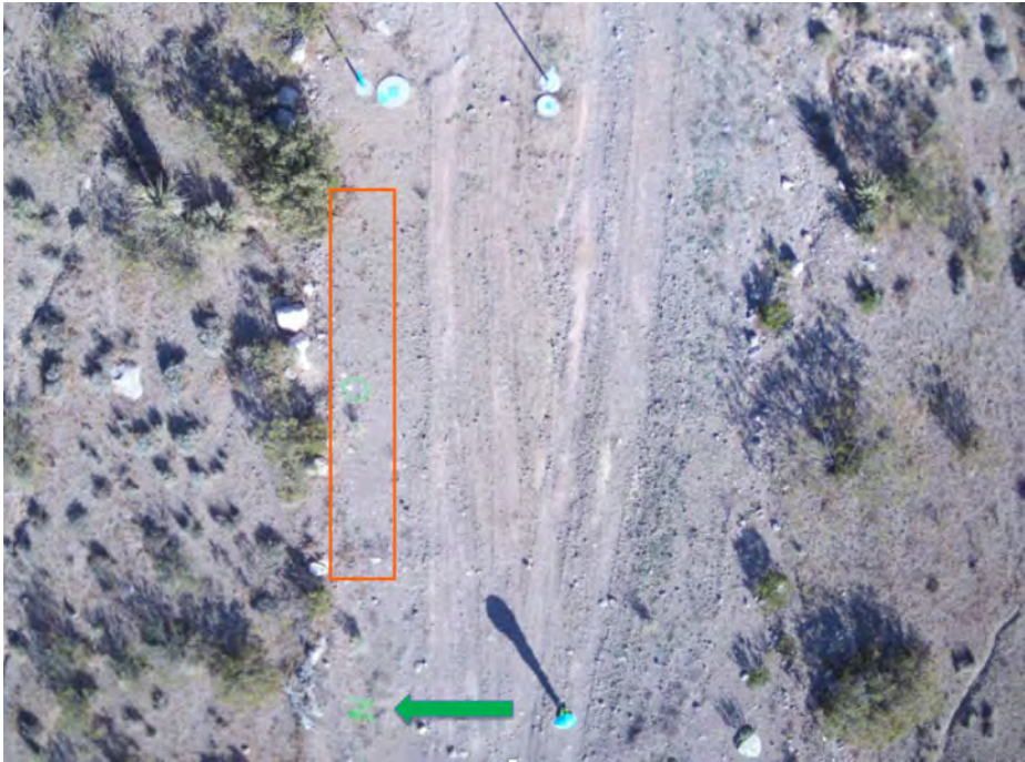
Figure 18A. Visual aerial image showing the location (orange box) of the temperature anomaly observed early morning on May 27, 2019. The water pipeline runs along the left side of dirt road, in the area of the orange box. The arrow points to the green “N” on the ground to help locate the area of interest in the visual and thermal images.
