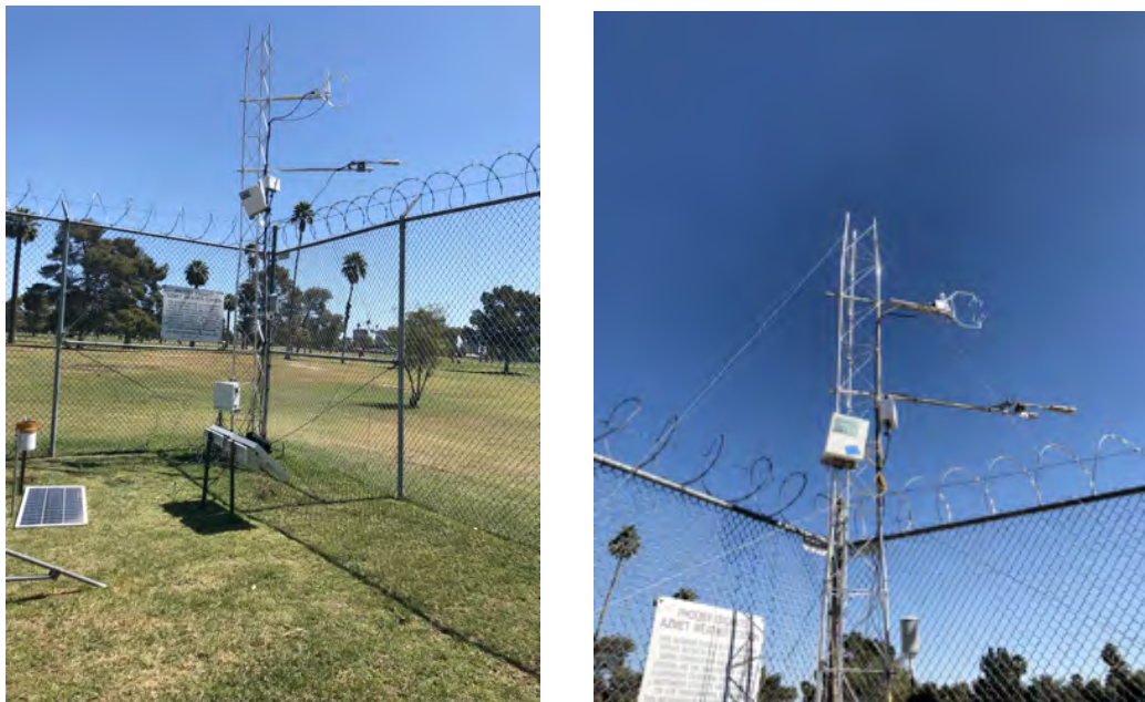
Figure 15. Photograph of complete eddy covariance system (left) that includes sonic anemometer, infrared gas analyzer, net radiometer, rain gauge, datalogger, soil moisture sensors, thermocouple sensors and solar panels. Primary instruments for eddy covariance system (right).
