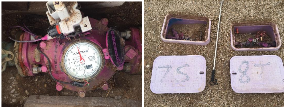
Obtaining flow rates for a tree and a shrub zone (valves on the right) from the dedicated water meter (left).
