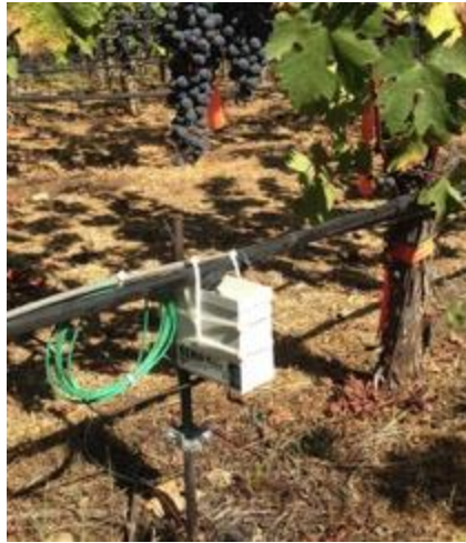
FIGURE 5: IRRIGATION GAUGE INSTALLED AT EACH SMART POINT
