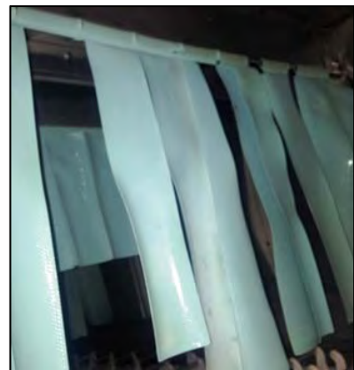
Figure 71: Missing strip curtains
