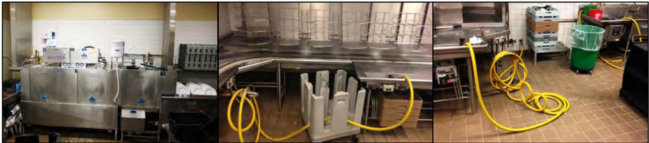
Figure 51: Dishroom pictures from left (dishwasher outlet) to right (pre-rinse station)
