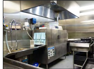
Figure 26: Heritage dishwasher and pre-rinse sink
