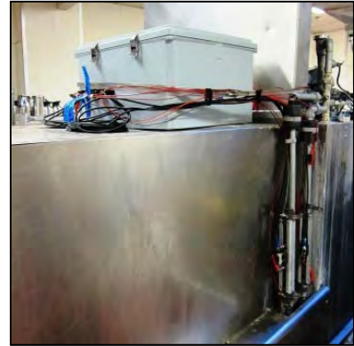
Figure 86: Instrumentation box and ultrasonic water meter transducers
