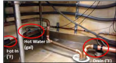
Figure 55: One water meter and two temperature sensor locations
