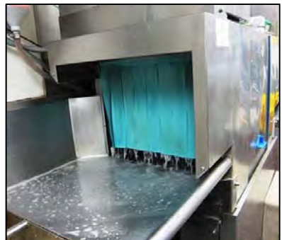
Figure 22: Overspray on inlet side slopping to pre-rinse sink
