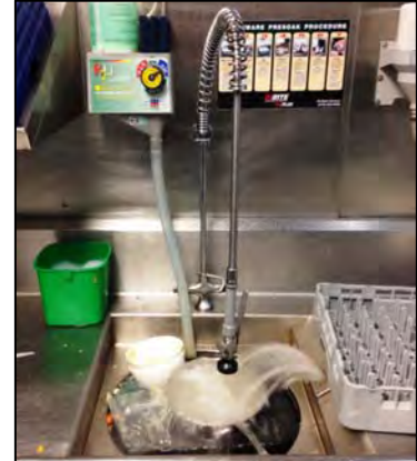
Figure 28: Hot water hose used to heat cold scrapper water
