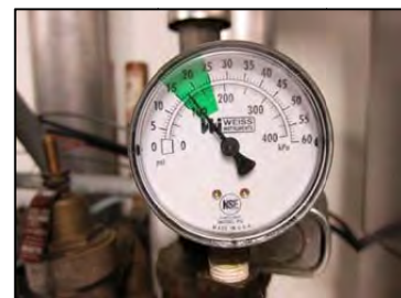
Figure 18: Original pressure gauge setting of 18 psi
