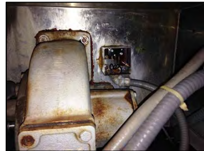
Figure 44: Tank fill relay switch
