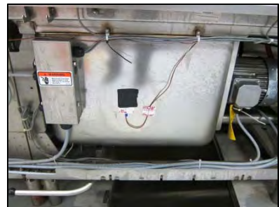
Figure 75: Temperature sensor affixed to tank
