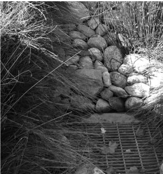
Once a year the grate to this catch basin should be lifted and the debris and sediment scooped out.
