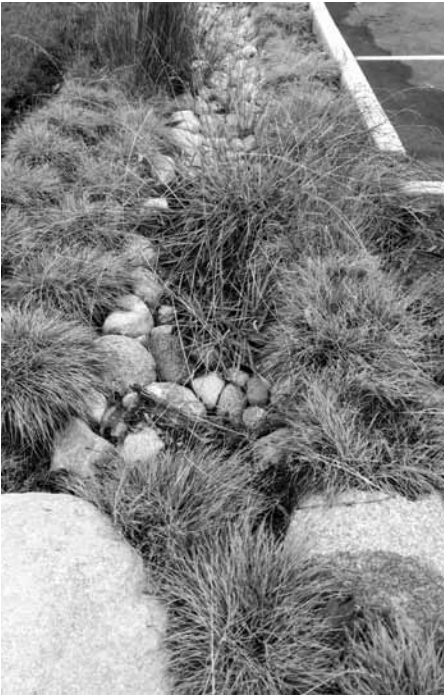
A colony of crabgrass has taken root in this rocky swale. If not removed, the crabgrass might affect the flow of water and cause unwanted pooling elsewhere.
